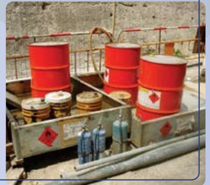
Provision of drip trays for chemical storage 化學品儲存器加設防溢盛器
