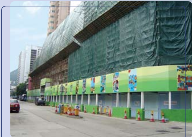
Recyclable metal hoarding and covered walkway 可循環再用的金屬圍板和有蓋行人道
