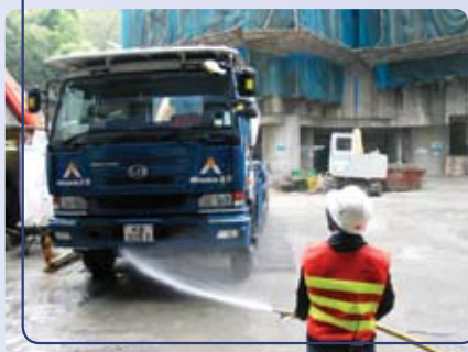
Recycled water for wheel washing of construction vehicles 以循環再用水清洗工程車輛輪胎
